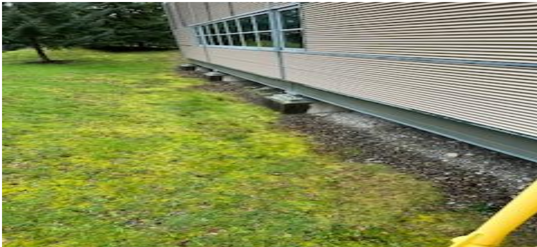
Side view of Washington EOC building showing steel-braced resting on framed base isolation foundation. Photo courtesy of Craig Johnson (NG7N).
