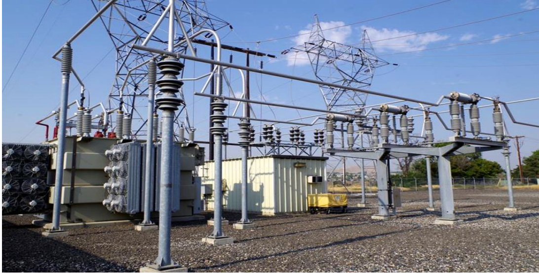
Typical Power Substation operated by Bonnaville Power, located in Richland WA.
